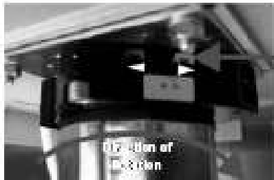
Limit Cover removed
